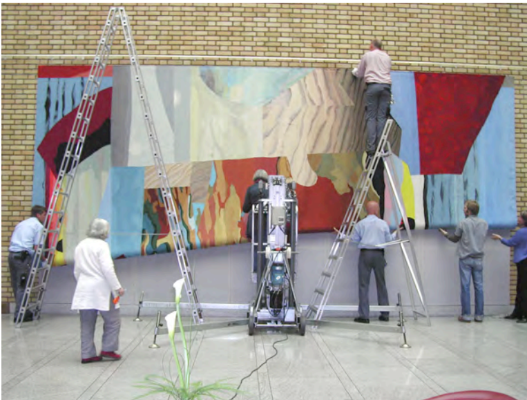
Completed in 2005, Blystad wove the "Landscape" tapestries in billedvev technique. 380x1500 cm. Here, workers are installing two of the three large panels in the Rambler's Hall (Vandrehallen) in the Norwegian parliament building.
